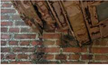
Dry rot in the roof ridges and deposits in the joints
