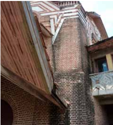
Deposits on the brickwork
