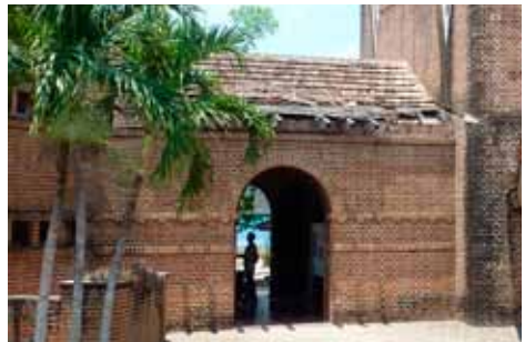
Decayed wooden roof ridges
