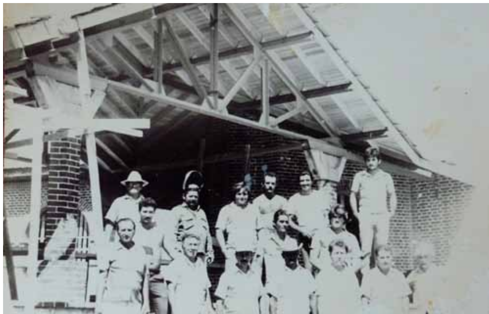
A group of builders/villagers poses in front of the building under construction, circa 1975. Jorge Santana collection
