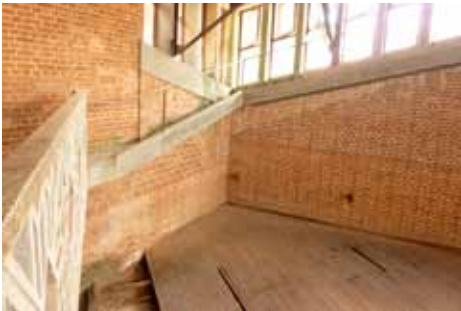
Rotten wooden floors in the dancehall
