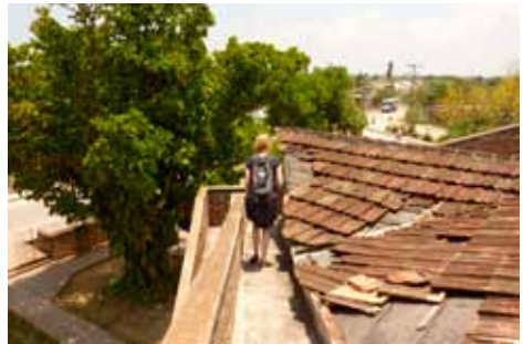
Broken and missing roof tiles
