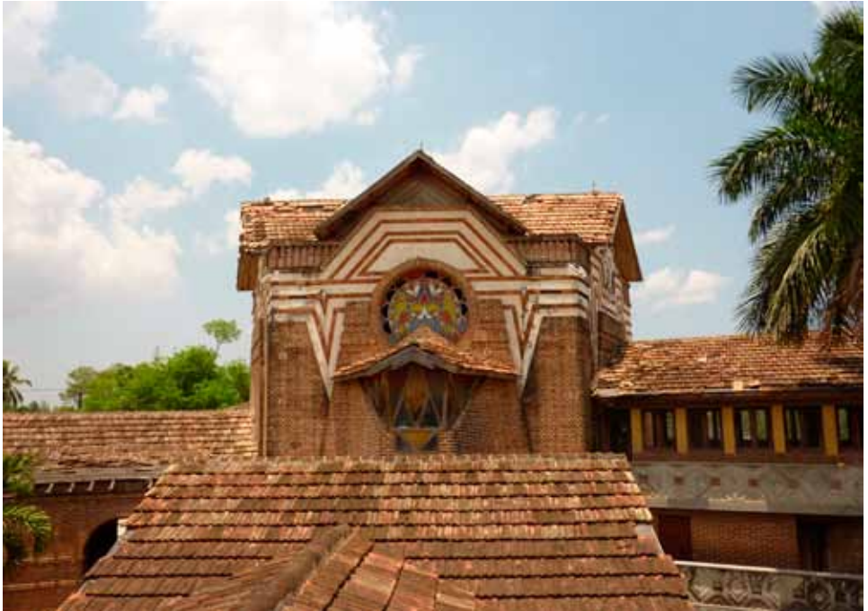
Decay of the roof
